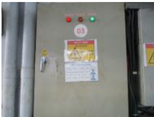
Safety signs on electric cabinet.JPG
