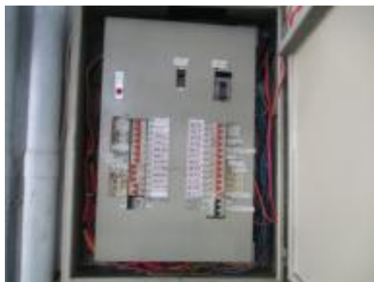
Electric panel with inner cover.JPG
