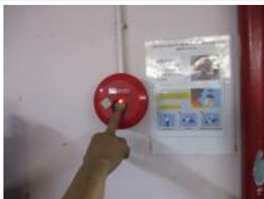
Fire emergency button.JPG
