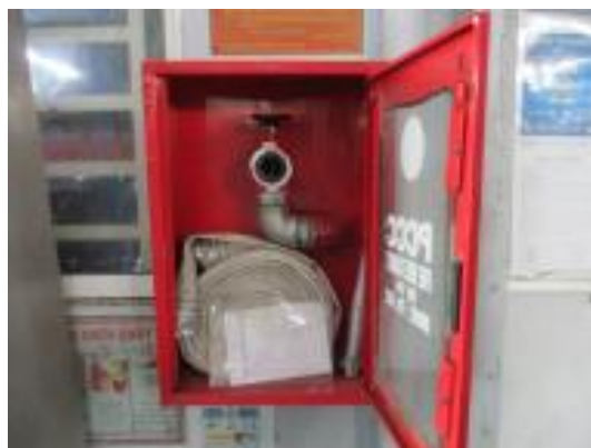
Fire hydrant and hose in cabinet.JPG
