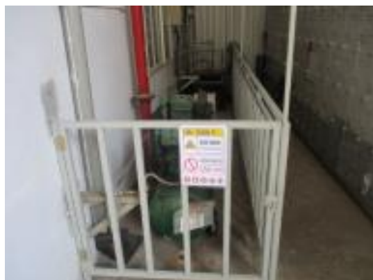
Air compressor station.JPG
