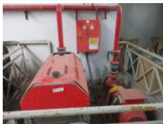
Fire pump station.JPG
