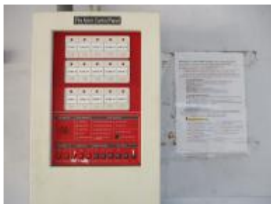
Fire alarm control panel.JPG
