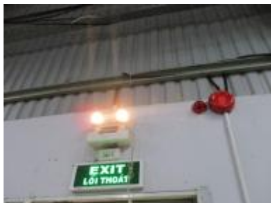
Exit light & sign.JPG
