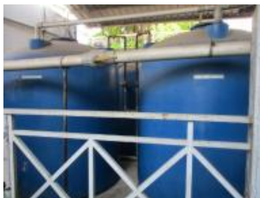
Wastewater treatment system.JPG
