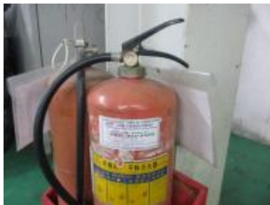
Fire extinguishers were maintained and recharged.JPG
